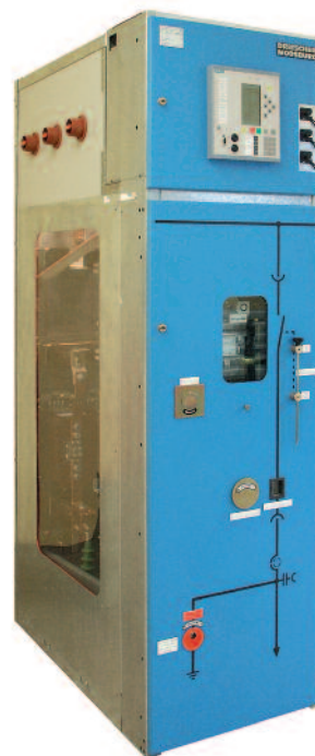
Fig. 3: 12 kV Circuit-breaker panel (WEL)
